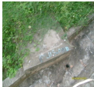
Fig. 3. Fix manhole under which the sink pipe passes to end in the catch basin
