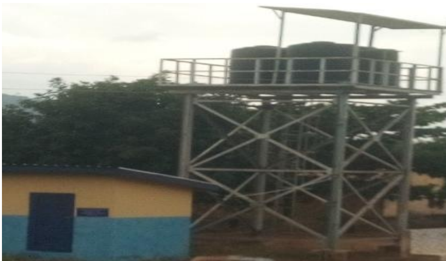
Fig. 7. Solar powered borehole in Itaogbolu
