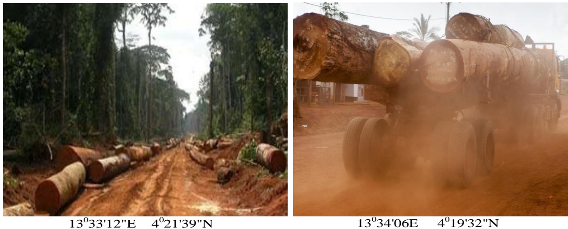
Fig. 7. Road construction within the forest for evacuation of timber Source: Field work, Council Forest Technical Unit and Getty View (2017)
