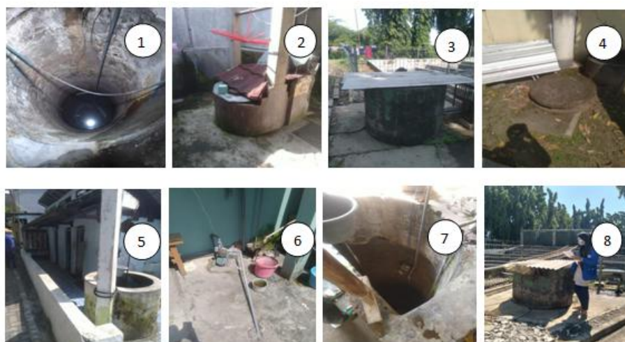
Fig. 8. The community well conditions
